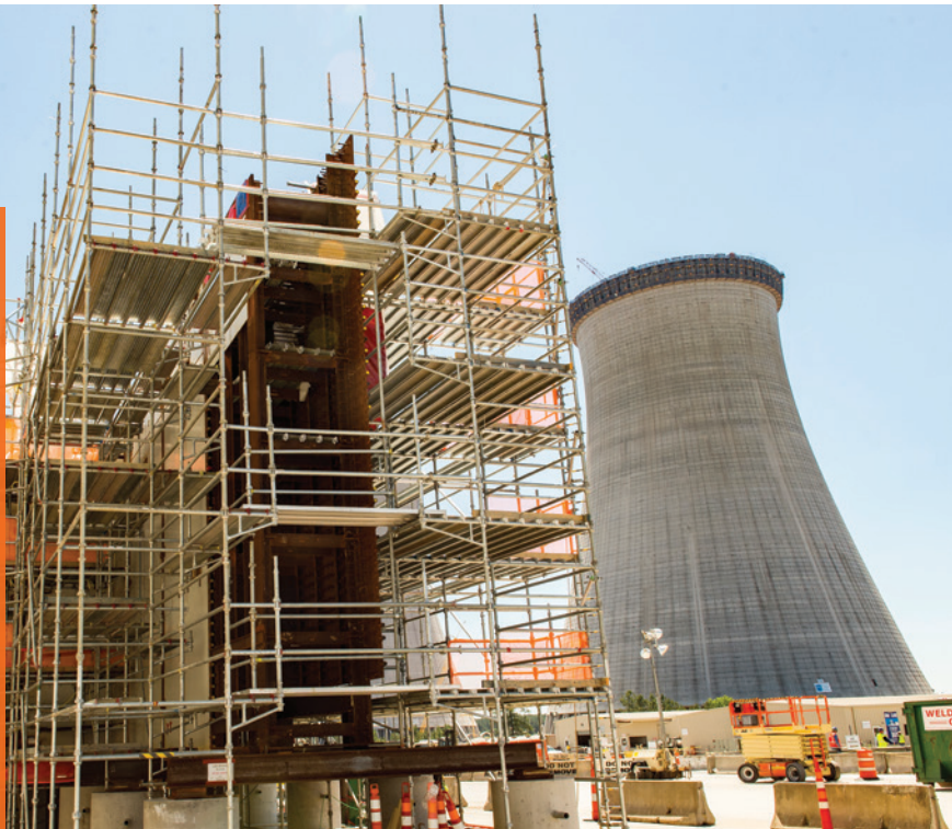
Georgia Power and its partners are building two nuclear reactors at the Vogtle Electric Generating Plant near Waynesboro, Ga.
